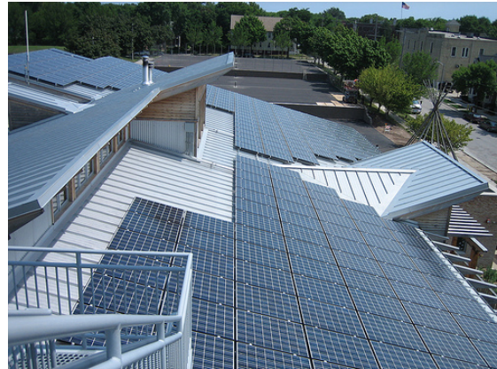
Rooftop solar panels used for energy production
