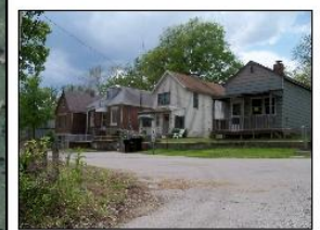
D - North of Rock Road, between Normandy High School and Lulu Avenue: These blocks contain 1.5-story, single-family homes. Many of these homes are showing signs of deterioration, and there are numerous vacant lots.
